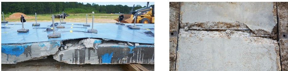
Figure 7: Intermediate crack-induced debonding (left) and concrete crushing (right) in the FT2 field test specimen.
